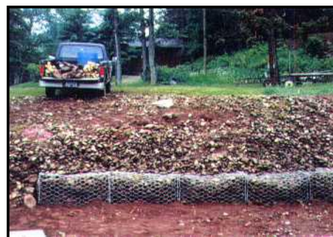
Gabion basket wall protecting an eroding shoreline. Top: before construction; Bottom: after installation. (Photos courtesy MN Board of Water and Soil Resources)
