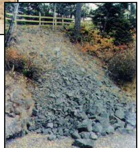
Critically eroded Lake Superior bluff. Top: before construction; Bottom: after using rock-fill method to remediate. (Photos courtesy MN Board of Water and Soil Resources)
